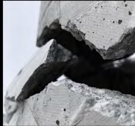
Wire infrastructure held together large portions of concrete
